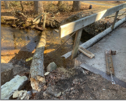
Fallen ash tree and damage to bridge Photo: Frank Lyter
